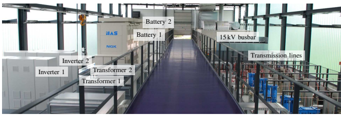
Fig. 2. Technology center of Younicos AG in Berlin with NaS Batteries, 500 kW inverters, transformers, transmission lines and 15 kV busbar.
