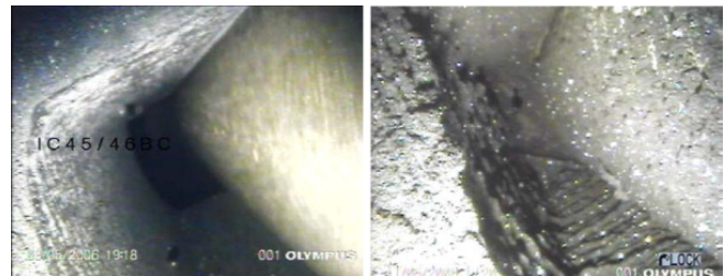
Figure 2. Tube support plate clogging: top view of a clean flow hole on the left side and an entirely blocked flow hole on the right side [9].
