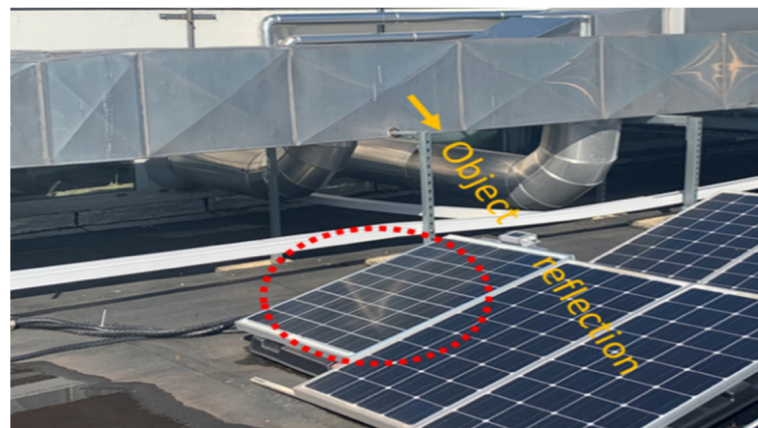
Figure 7. Over-illumination effect (circled in red) on the PV panel.
