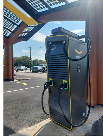
(b) Fastned charging point
